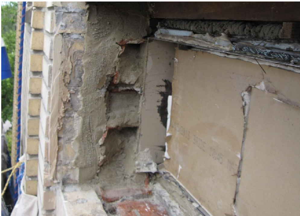
figure no.11: Next...the broken terracotta block is filled with mortar so that we can get a good bond with the new inside wall.
