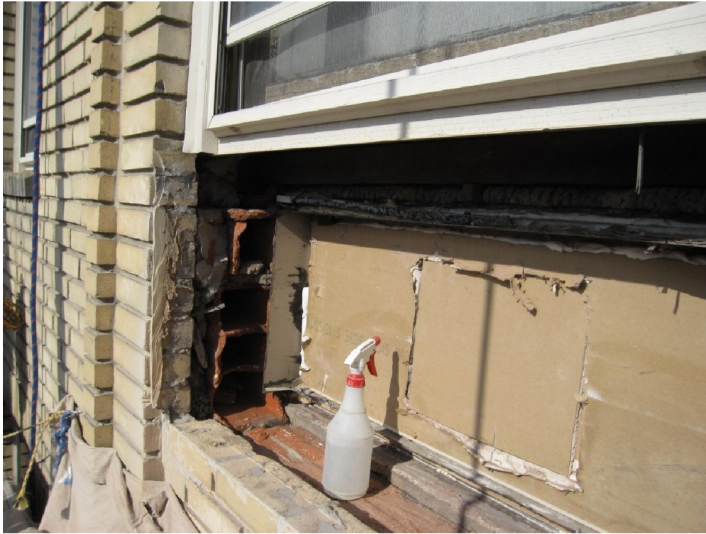
figure no.10: This picture is from Unit F4 after the debris has been cleaned up. You can see remnants of the old A/C sleeve that was abandoned in place. Abandoning a sleeve in place provides a path for water infiltration. In a driving rain the water could travel along the sleeve and find its way to the concrete slab, under the floor, and travel until it finds a path to drain. With the old sleeve cut back we now have room to rebuild the inside wall.
