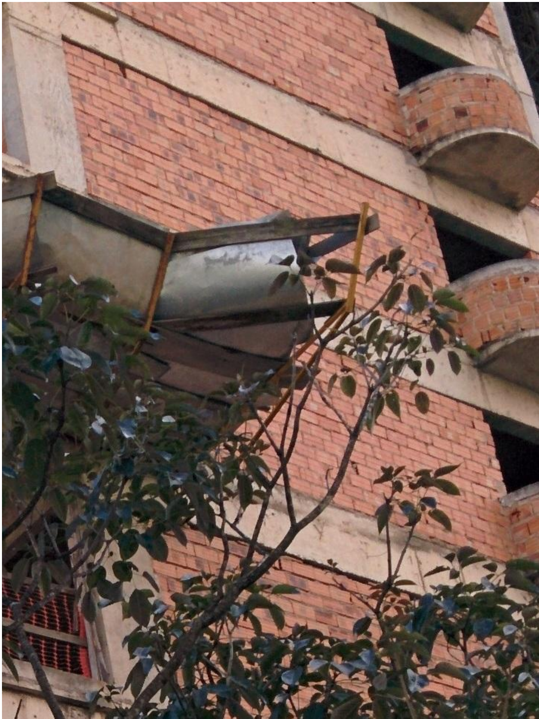
figure no.4: Example of steel reinforced concrete column and beam construction before the brick façade is added.
