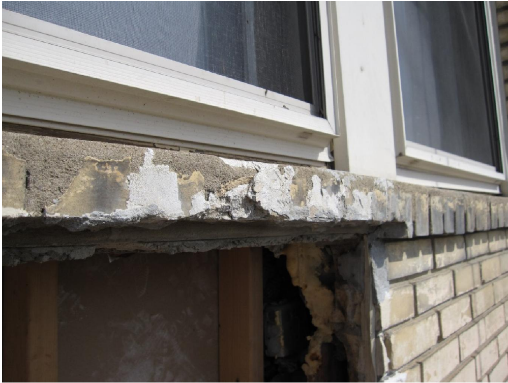
figure no.8: This is a picture of a sill cap. It will give you a good idea of the kind a masonry work that has been done by past air conditioning contractors.
