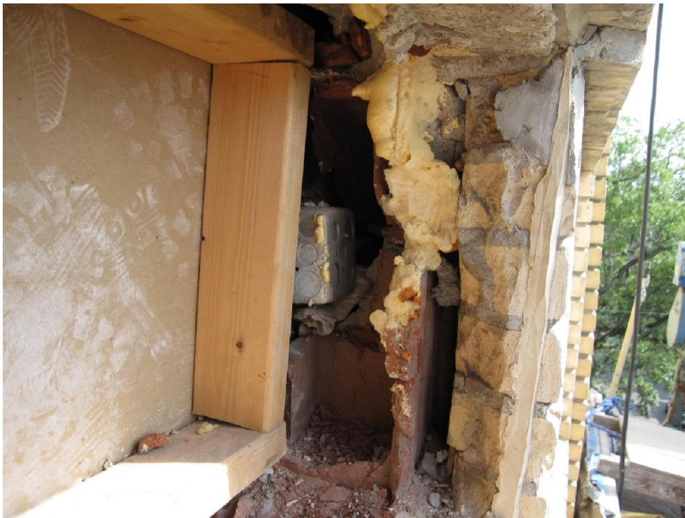
figure no.9: You can see that the inside terracotta block was not cut, but broken out to make room for the sleeve. The next step is to clean the debris that was left behind from the previous air conditioning contractor.
