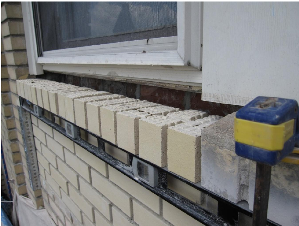
figure no.15: The sill cap course of brick is set in place. Notice that each brick in the sill cap is scored to help bind the mortar top coat to the course and to keep it from delaminating.
