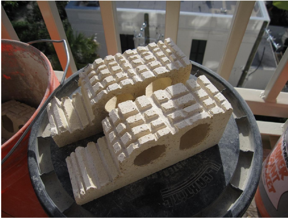
figure no.14: The brick for the sill cap is shortened, grooved and a web is removed to make room for the proper thickness of the mortar bed to support the window above.
