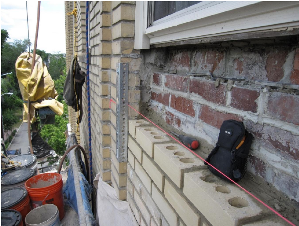
figure no.13: A temporary jig is installed to help guide setting the outside brick in the correct place.
