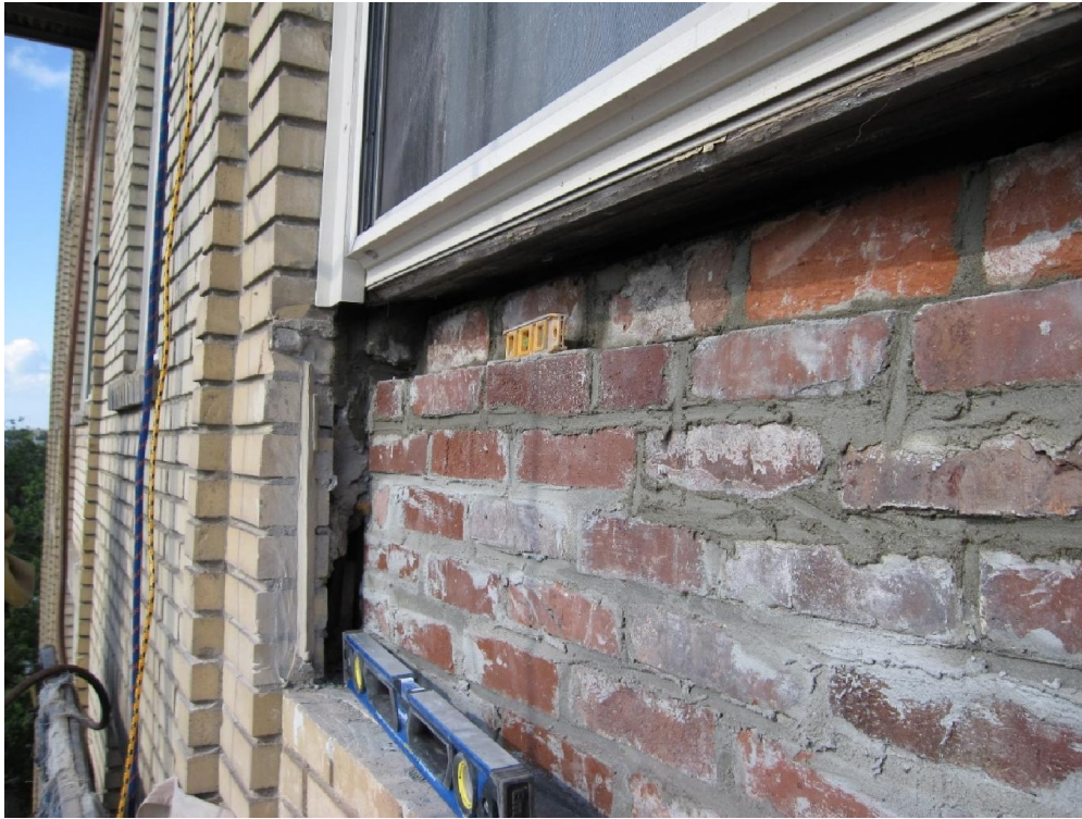
figure no.12: A new inside wall is built to replace the missing terracotta section. The new inside wall goes all the way up to support the window. We have found that none the air conditioner openings have lintels installed over the sleeve. A lintel is a steel angle iron that carries the load above.
